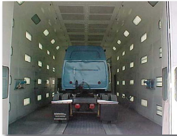
This truck paint spray booth at Midway, Inc. in Monroeville eliminates pollutants from the air and helps the autobody shop comply with federal Clean Air Act standards with financing through OAQDA's Clean Air Resource Center.
