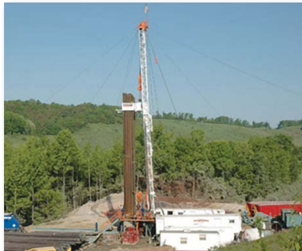
This drilling rig in Tuscarawas County was constructed with funds from an Ohio Coal Development Office grant in 2007 to The Ohio State University. Researchers there explored the production of hydrogen from coal and a stream of carbon dioxide suitable for underground sequestration.
