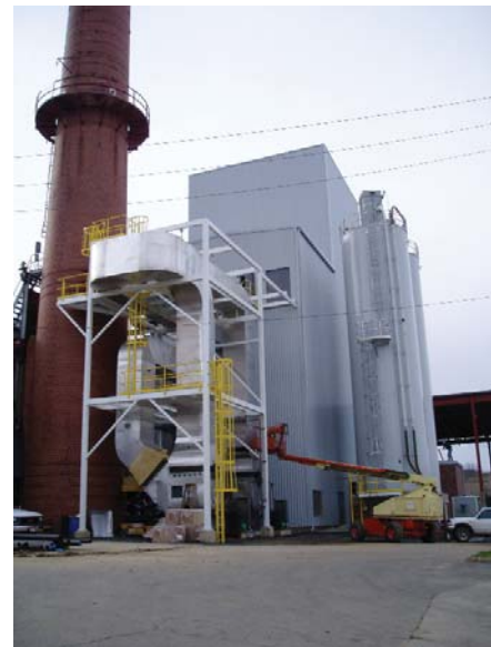
This humidity and ethylene management equipment utilizing Sorbitech technology for commercial refrigeration systems at Ohio University was constructed with funding from OAQDA as part of a project to improve air quality throughout the institution.
