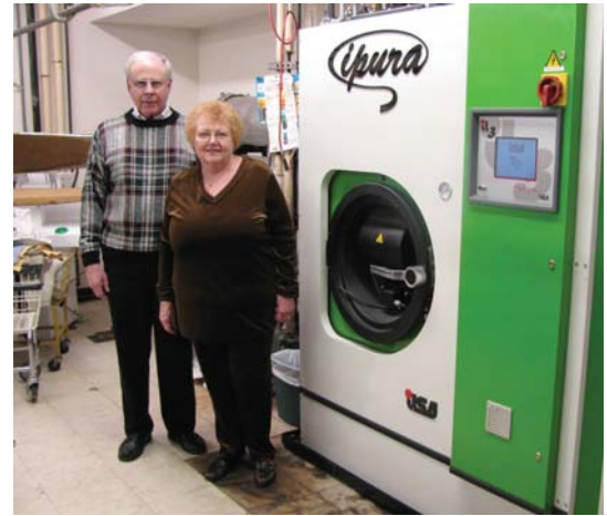
Jim and Linda Lucas, owners of Highlander Dry Cleaning in Newark, stand near new equipment purchased with financing from OAQDA's CARC. The new machine reduces emissions and helps them comply with clean air mandates.
